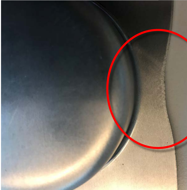
“in-plane crack” Outer line shear crack (tendency) ?
